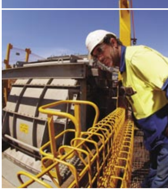
Head Chute, Dampier Port Upgrade
